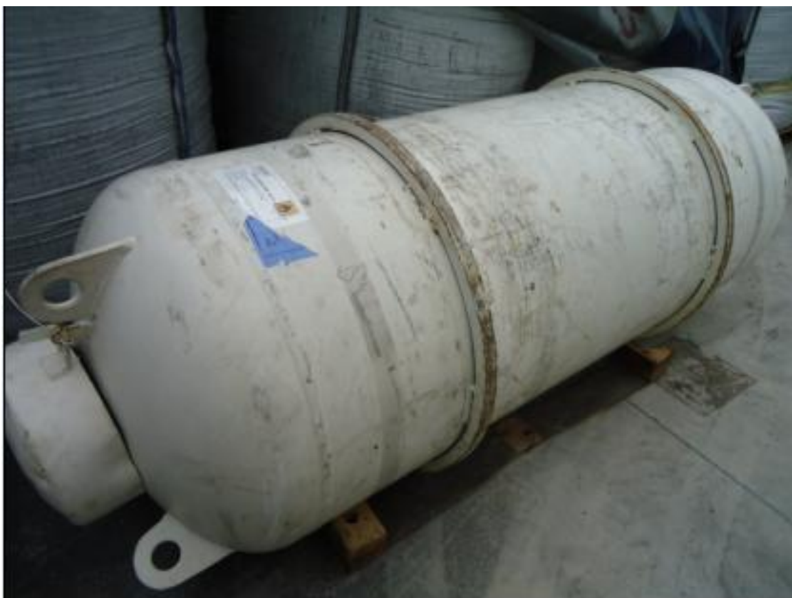
Picture 3- The whole gas tank
